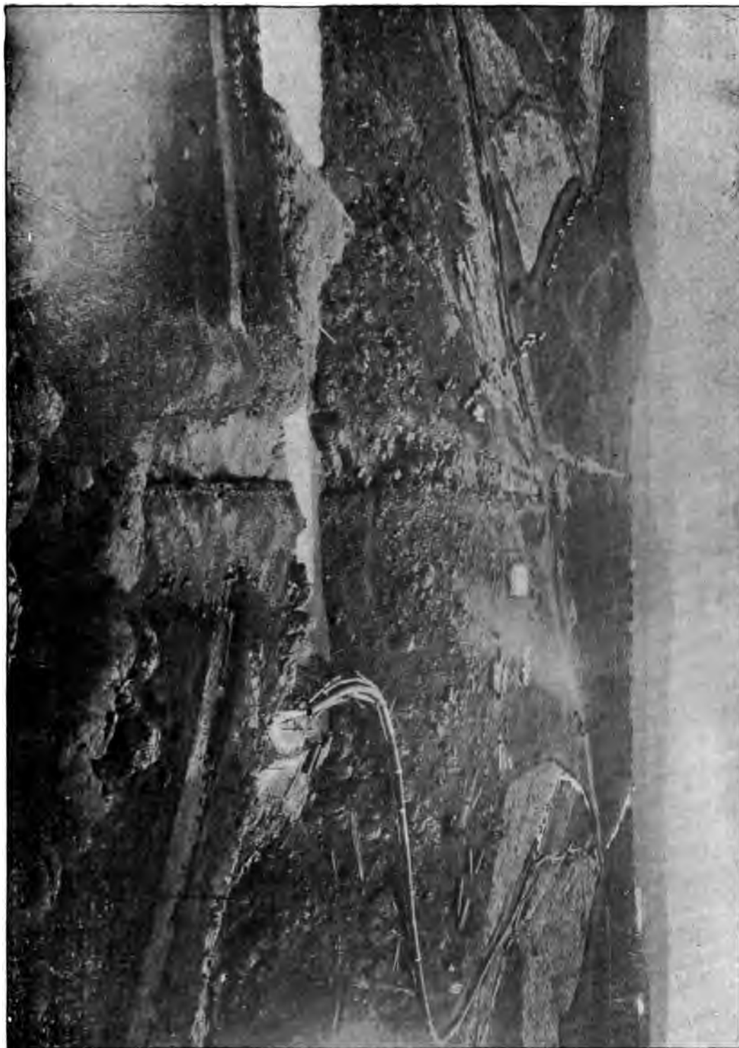
BEGINNING THE CONSTRUCTION OF LA MESA DAM. (From "Eighteenth Annual Report of U. S. Geological Survey.")
