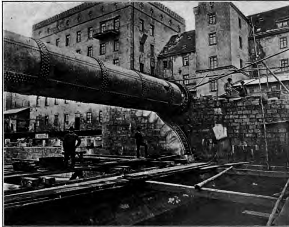
ROLLING DAM AT SCHWEINFURT, GERMANY. THE ROLLER RAISED.
