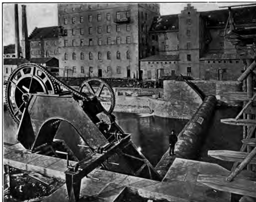
ROLLING DAM AT SCHWEINFURT, GERMANY. THE ROLLER LOWERED.
