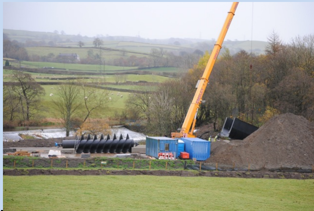
Archimedes' screw systems have already been implemented throughout the UK, as pictured, and Europe. New England Hydropower is now bringing this ancient technology to the Northeast. (Photo credit: Chris Conover)
