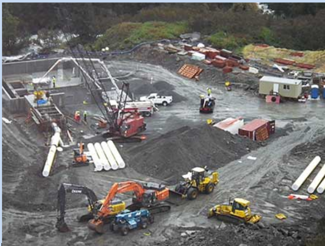
Allison Creek Hydropower Project near Valdez. Construction of Powerhouse and Penstock. Photo: M.D. Miller Taken Sept. 15, 2014.
