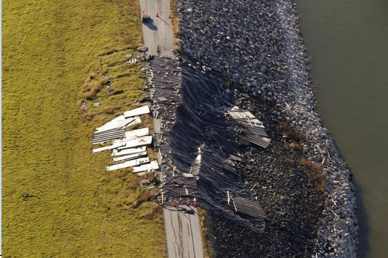
Nathan Hunsinger/Staff Photographer Tarps weighted down by sandbags are covering the 160-foot-long landslide that stretches along a section of the Lewisville Lake Dam. Repairs had been planned for Monday, but those plans may be jeopardized by rising lake levels.
