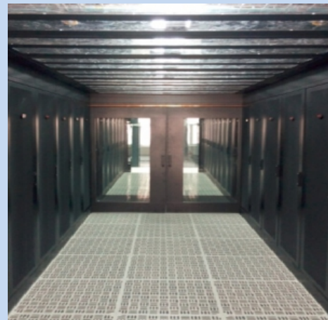
Data center cold aisle
