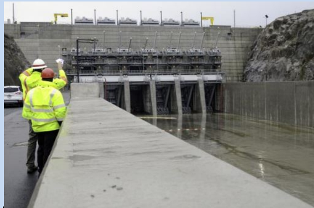
Each of these six spillway gates are 50 feet lower than those of the main dam, allowing water to be released earlier in the event of heavy rains.
