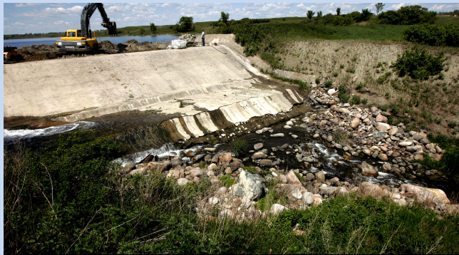
In this Grand Forks Herald file photo from June 2008 construction workers repair of Tolna Dam using Bentomite Clay to repair seepage that was causing leaks for the previous five years. Grand Forks Herald file photo.
