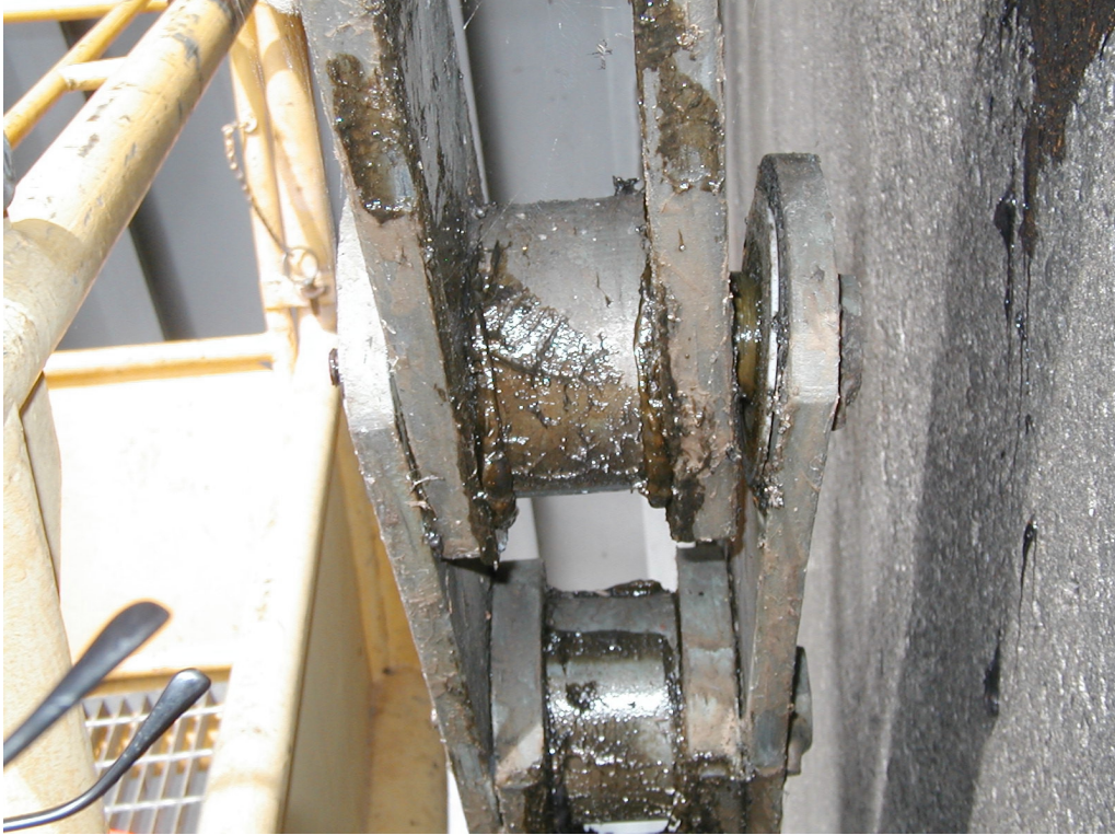
Photo 1: Wanapum Dam, Tainter Gate 1, left bank hoist chain bent side bar
