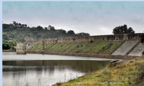
The Roman dam at Cornalvo in Spain has been in use for almost two millennia. Credit: Wikipedia/ CC BY-SA 2.0
