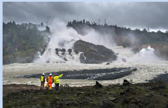
Workers and a firefighter watch water pouring down Oroville Dam's damaged main spillway on Feb. 20. Hector Amezcua hamezcua@sacbee.com
