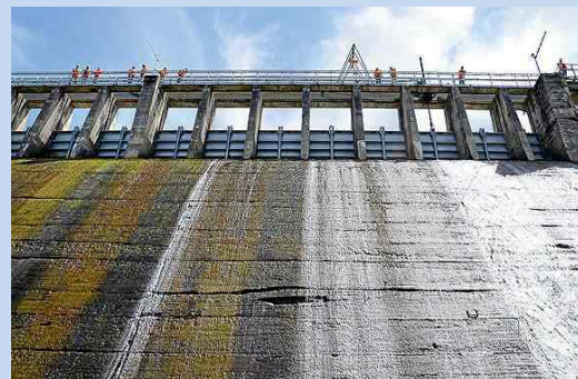
The Scott Dam of Pacific Gas and Electric Co.'s Potter Valley Project is set to go under review for relicensing in 2022 by the Federal Energy Regulator Commission. Justine Frederiksen — Ukiah Daily Journal
